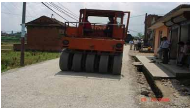
Photograph 7. Rolling process being carried out by a pneumatic tyre roller from edge to centre
