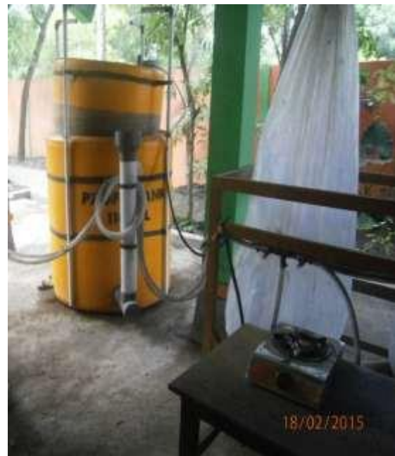
Figure 4 Anaerobic Digester with Wet Fermentation of Food Waste
