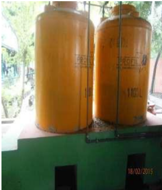
Figure 3 Anaerobic Digester with Dry Fermentation
