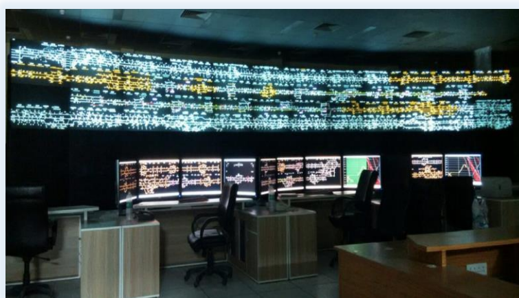
Figure 3: Operations control centre Tundla, North Central Railway
